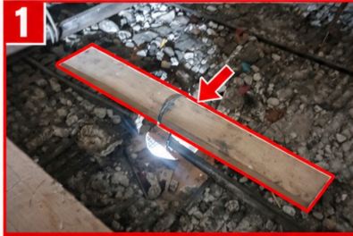
MAKESHIFT LUMBER ACCESS OVER THE HISTORIC CEILING.
