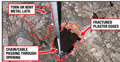
2 TORN OR BENT METAL LATH AND FRACTURED PLASTER AROUND RIGGING PENETRATION.
