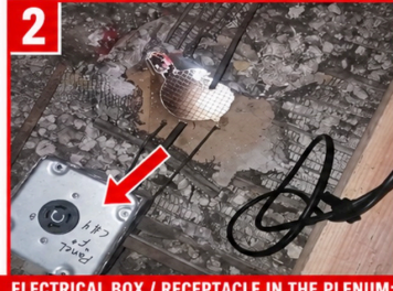
ELECTRICAL BOX / RECEPTACLE IN THE PLENUM; OWNER REPORTS NO ELECTRICAL, PERMIT. PHASE CANNOT BE DETERMINED FROM THIS PHOTO.
