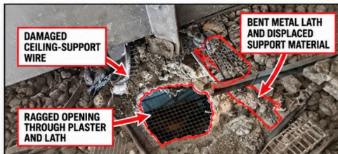
3 CHAIN/CABLE AND HARDWARE PASS THROUGH DAMAGED CEILING OPENING.
