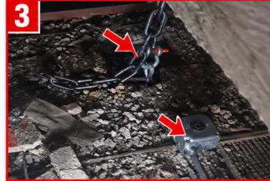
ELECTRICAL CABLING, RIGGING HARDWARE, AND CEILING DEBRIS IN THE SAME PLENUM AREA.
